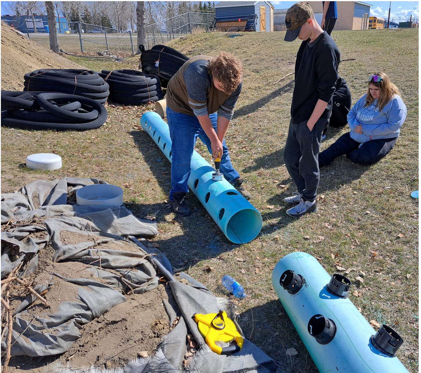
Above: Students building manifolds for the climate battery at the Strathmore High School Community Greenhouse.
